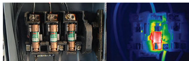
Thermal Image, Corroded Fuse
