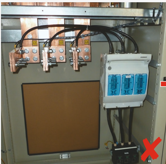
Before the intervention: The SPD installation fails to meet the condition as regards the length of supply conductors
